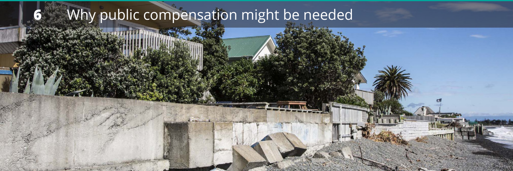
Severe coastal erosion at Haumoana
