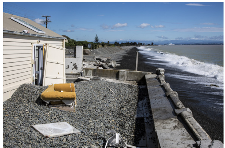
Coastal erosion damage at Haumoana
